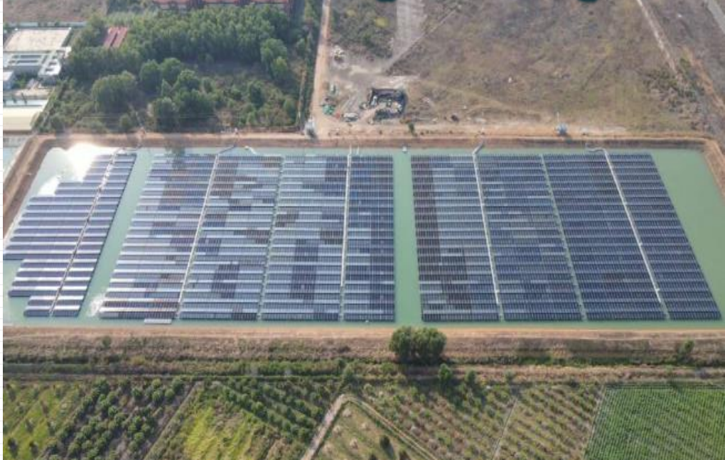
2023 Vietnam Phuoc dong 4MW Floating Solar
