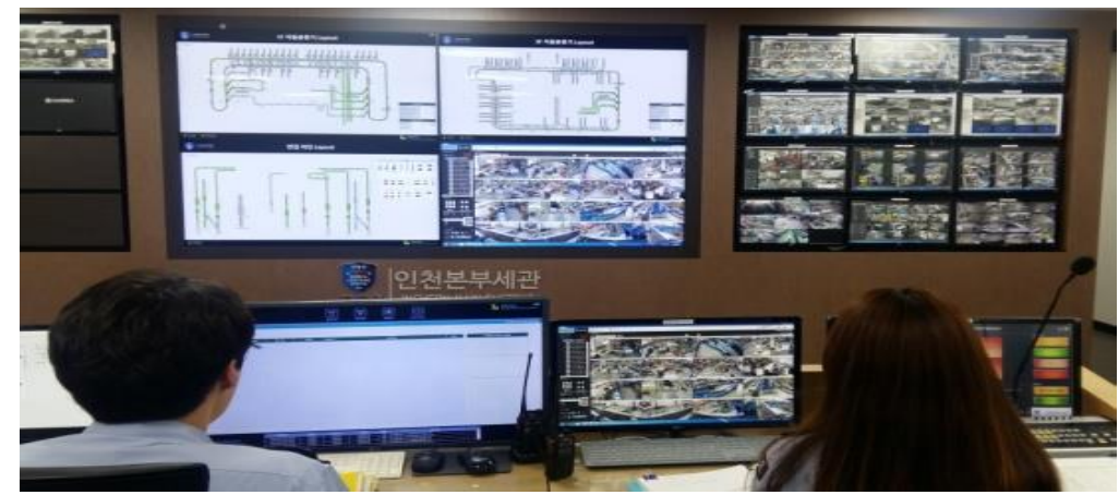
Integrated Control Room
