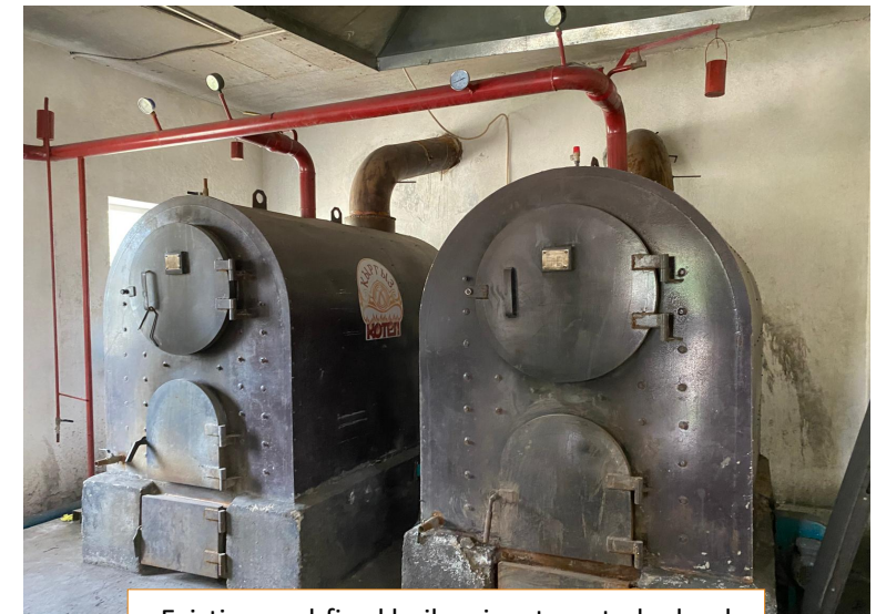
Existing coal-fired boilers in a targeted school
