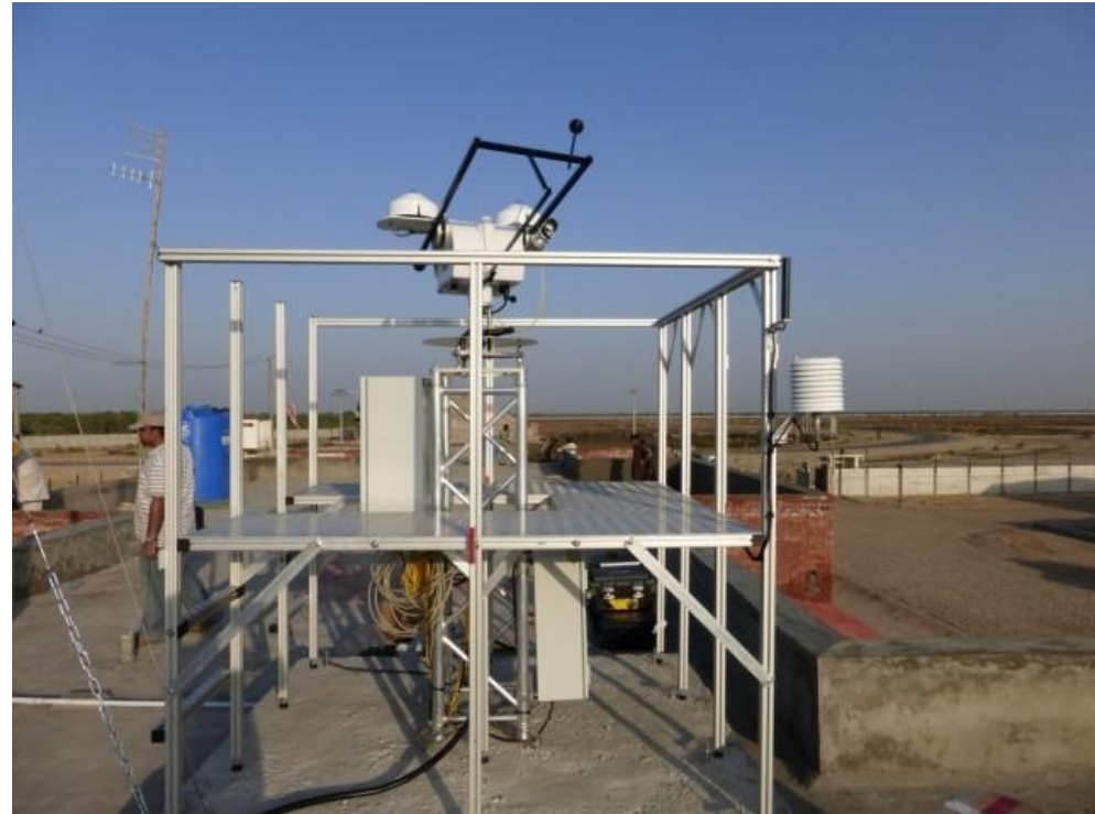
Quaid-e-Azam Solar Park, Bahawalpur
