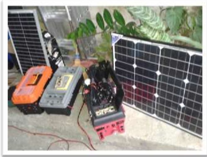
Solar PV Panels
