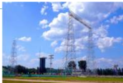
UHV DC Test Base (Changping, Beijing)
