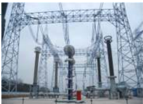
UHV AC Test Base (Wuhan)
