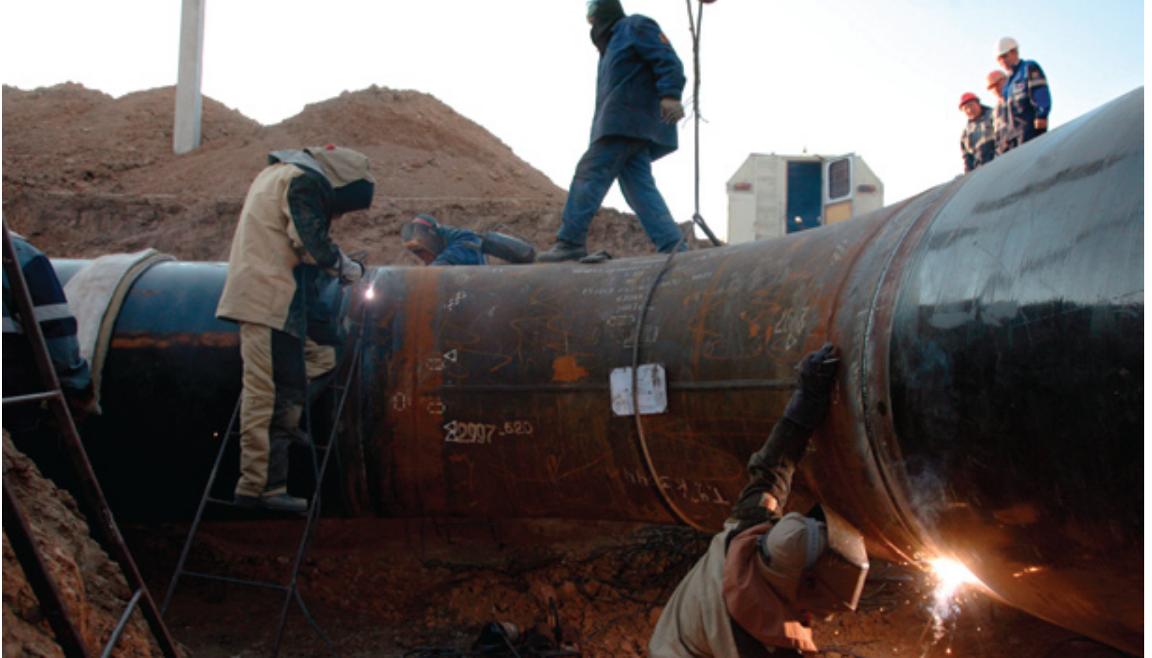
■ Gazprom welders work on a pipe during reconstruction works on the pipeline in Alexandrov Gai village at the border between Kazakhstan and the Russian Federation. The pipeline is expected to increase the possibilities of gas transport from Central Asia to Europe.
